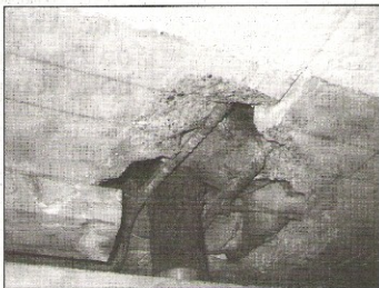
Exposed Reinforcing Rod and Corrosion
