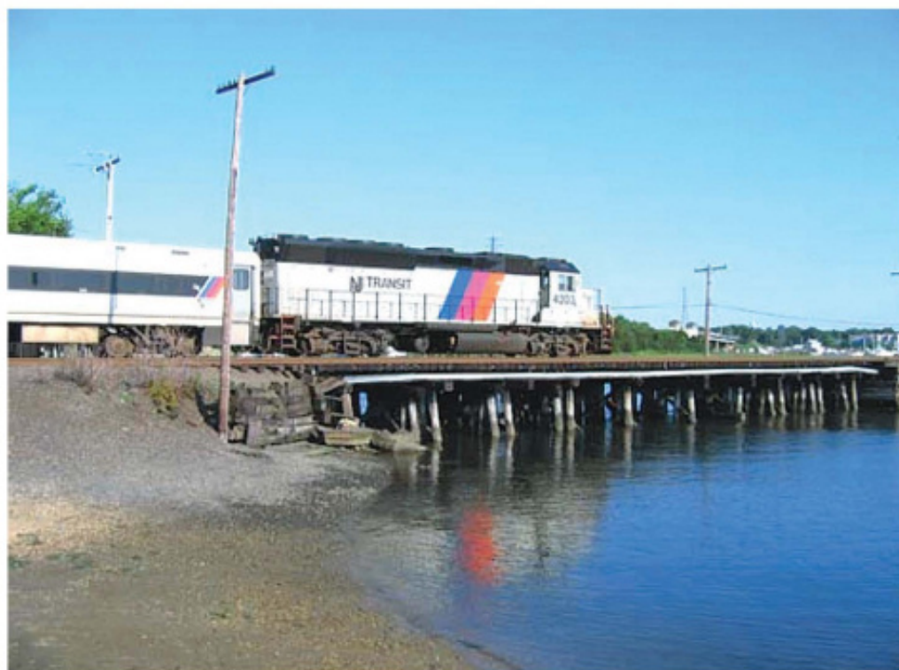
NJ Transit train rolls northbound across the old wooden bridge over the Manasquan River at low tide. The lagoon is in the near right.
