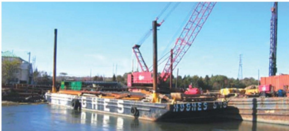
Barge blocks access to the bridge during construction.
