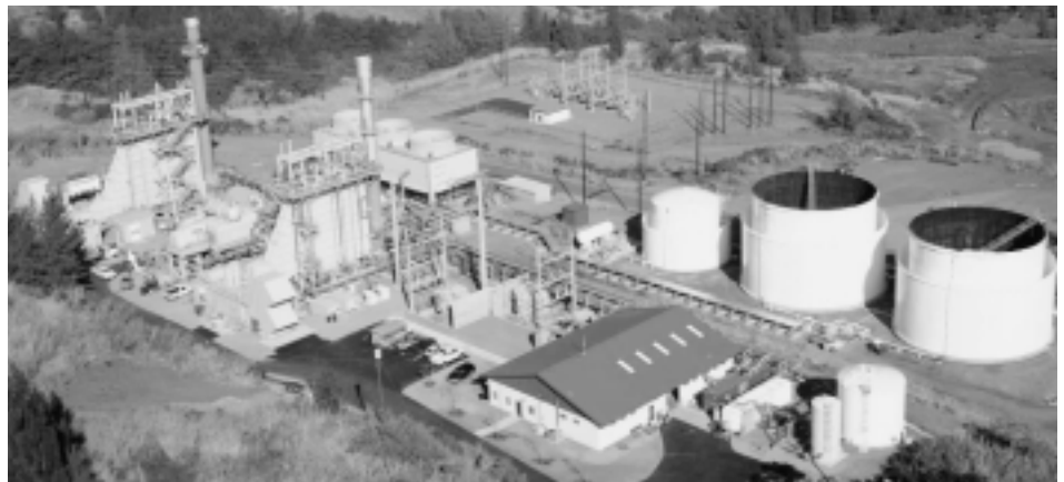
AES Hawaii New Cooling Tower Day 19 – Four Cells Completed and Ready for Operation. Fifth Cell was Completed on Day 21.
