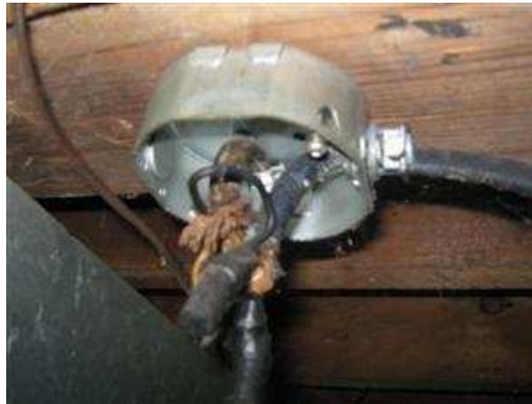
11.5 WIRING / CONDUCTORS Picture 1
