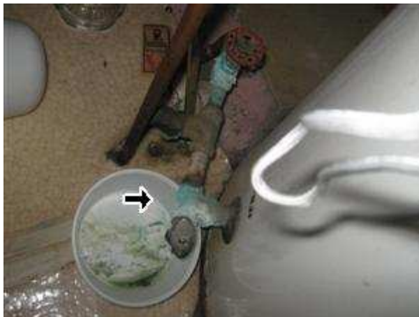
15.0 WATER HEATER Picture 1
