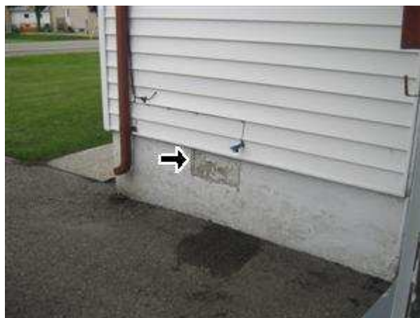
9.4 CRAWLSPACE VENTILATION Picture 1
