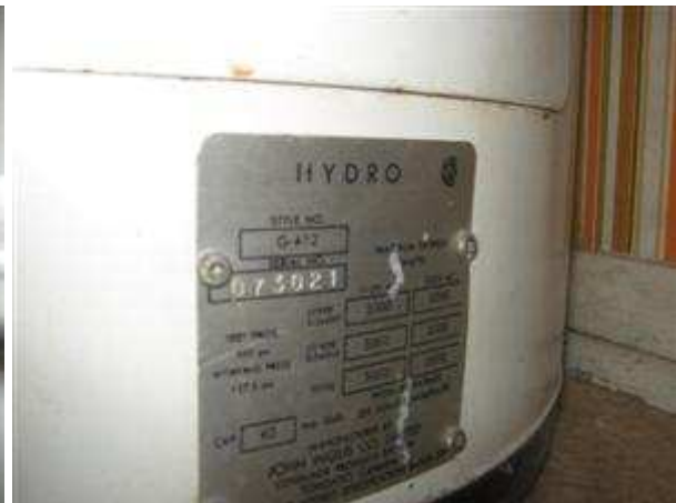
15.0 WATER HEATER Picture 2
